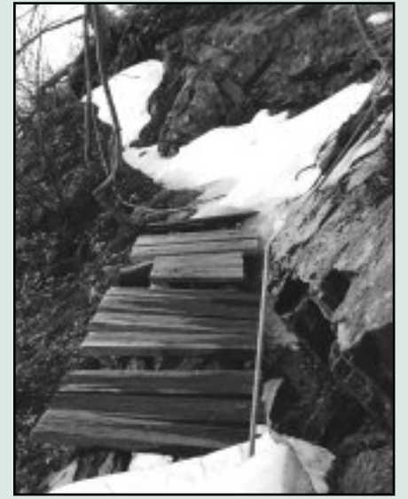
Among this season's projects: replacing this bridge on the Stillman Trail in Storm King State Park.
